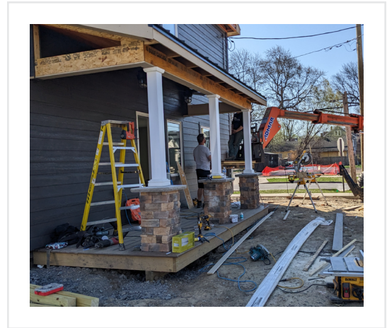
Members of Home HeadQuarters' construction crew at work on a new single-family construction project encompassing net-zero building and an expected PHIUS certification as part of the Syracuse Resurgent Neighborhoods Initiative.
